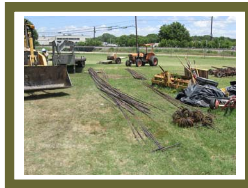
Equipment and supplies being used to build the new Golf Course Clubhouse.
