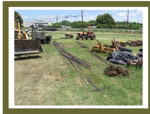
Equipment and supplies being used to build the new Golf Course Clubhouse.
